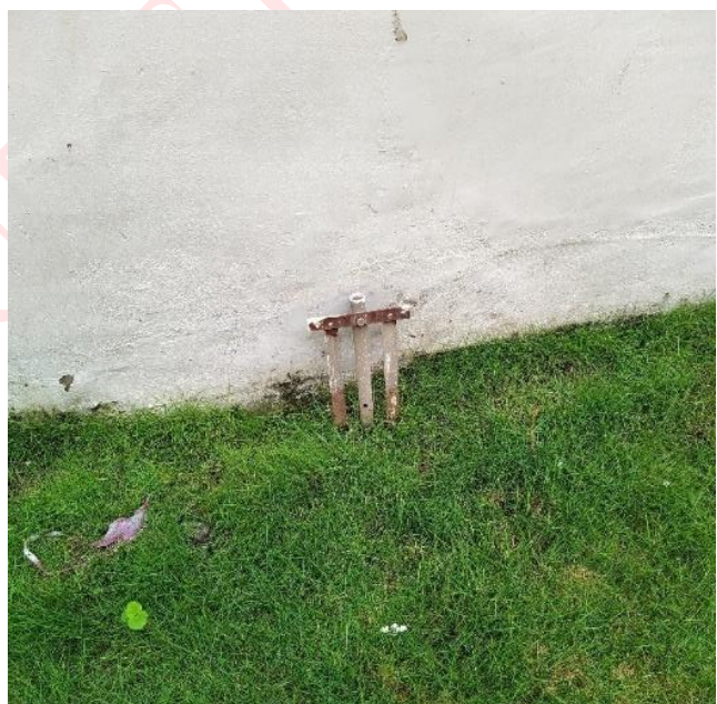
Figure 14 - Safety, electrical earthing compliance
