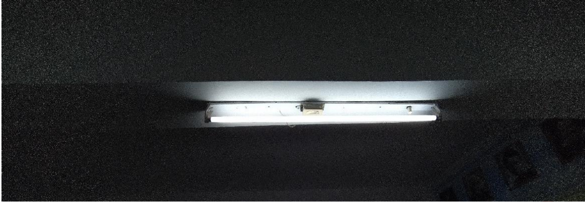
Figure 10 - T5 & T8 tube lights with Electromagnetic choke
