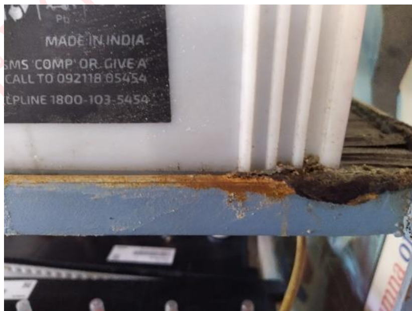
Figure 12 - Galvanic reaction causing damage to battery life.
