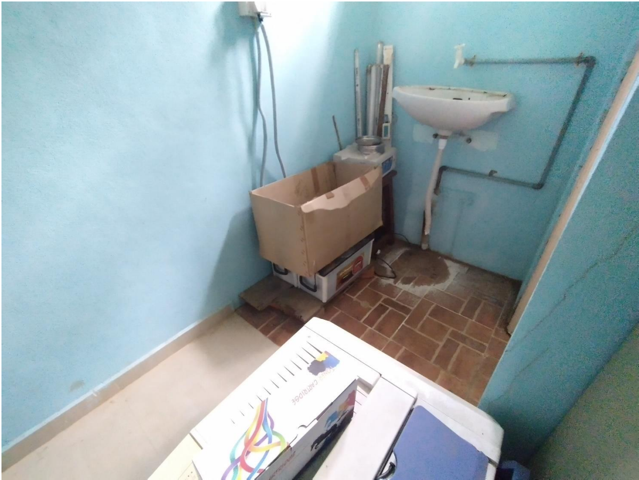
Figure 13 - Battery placement, Need cross ventilation.
