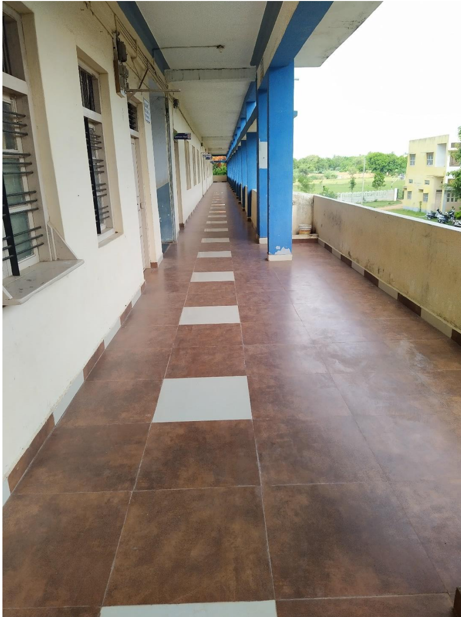
Figure 10 - absence of waste collection bins in the corridor
