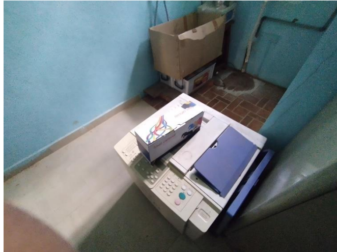
Figure 16 - Placement of battery without ventilation
