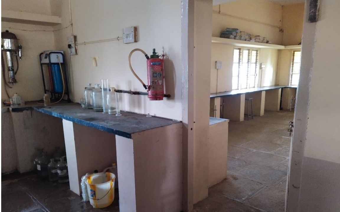
Figure 20 - No ready access to fire extinguisher.
