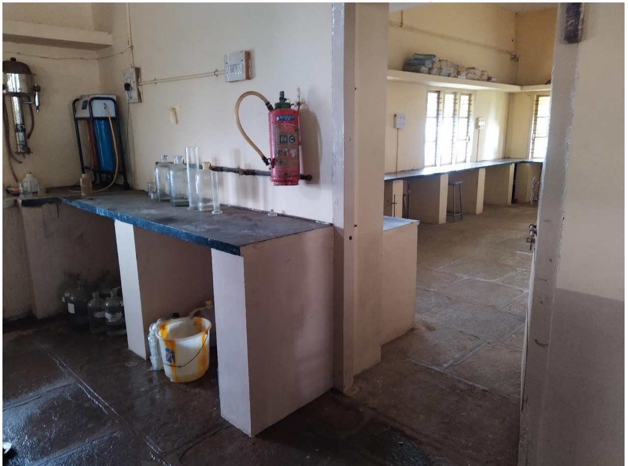
Figure 16 - Placement of Fire extinguisher.
